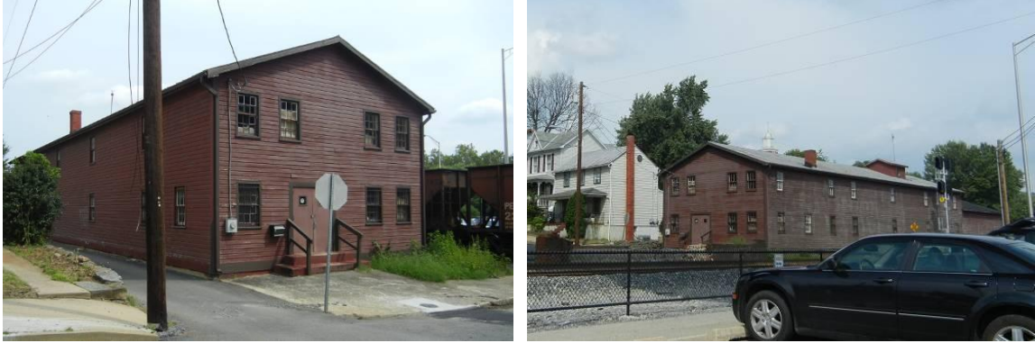
Figure 14 Warehouse on Virginia Ave (1 st Street). Notice how close the railroad track is to the structure as seen by the freight cars passing by on the right in the first image.
